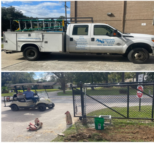
The middle school gate has been repaired and a remote operator has been installed.
